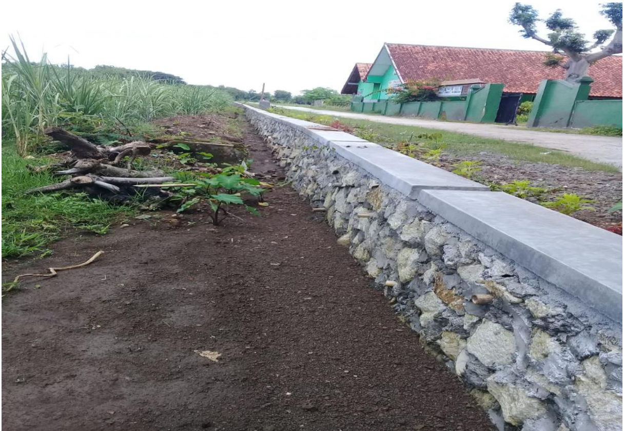
Gambar III.3 Talud Jalan Sengereng Argodadi
